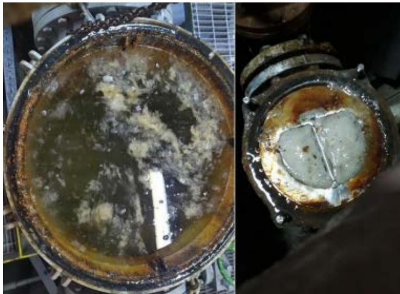
Figure 5. Seawater Inlet filters after mucilage effects [27].
