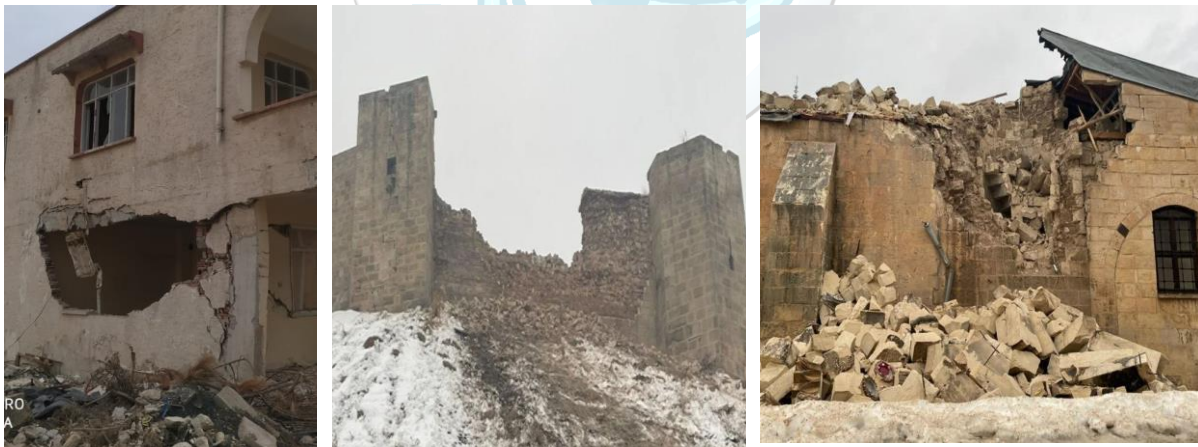
Figure 6. out-of-plane damages in masonry structures in the earthquake region [13]
