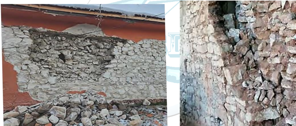
Figure 8. Poor masonry material properties in masonry structures in the earthquake region
