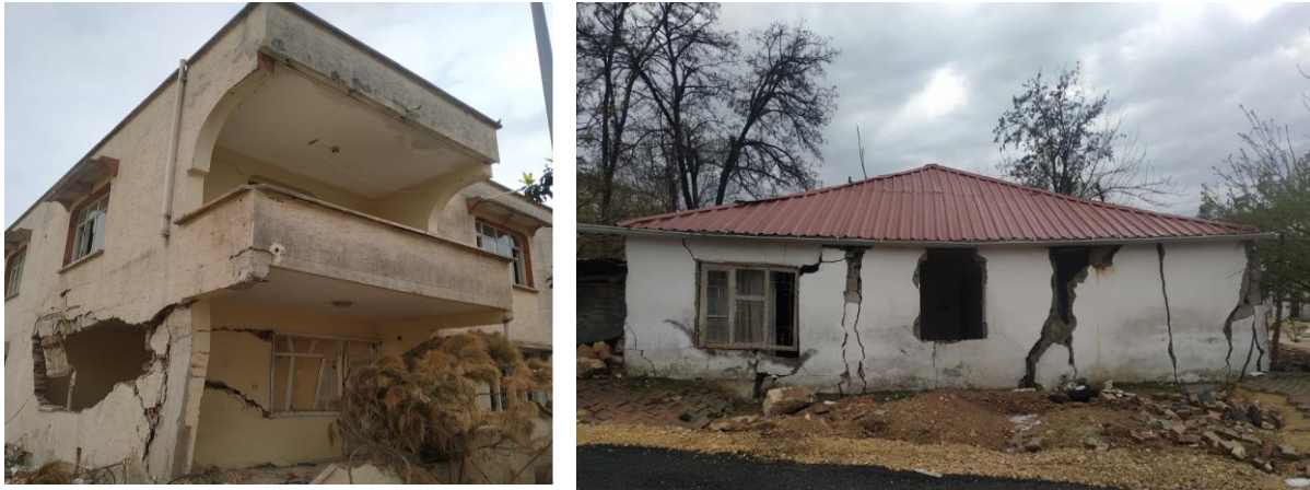
Figure 7. In-plane damages in masonry structures in the earthquake region
